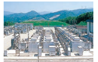
Harmonic Filter Equipment
