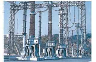
Capacitor Voltage Transformer
